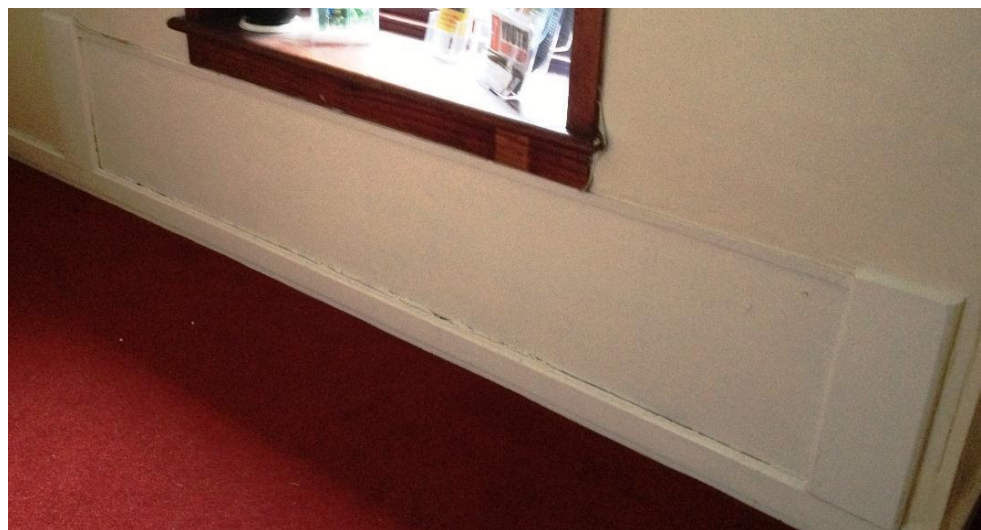
Figure 1: One of the unusual panel radiators - in the hall
