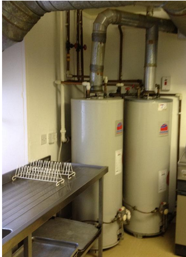
Figure 2: The existing Andrew's water heaters in the kitchen
