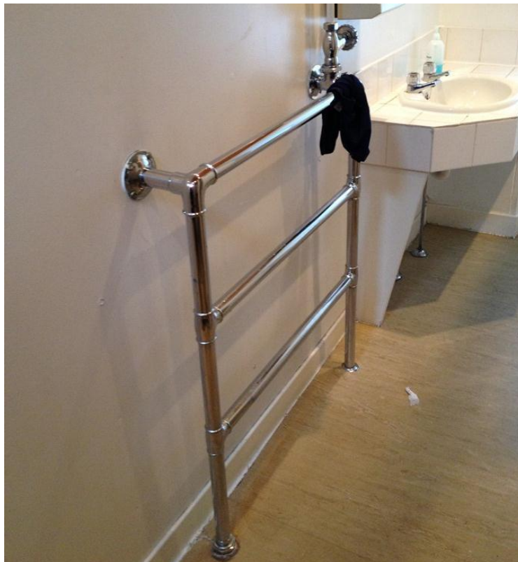
Figure 3: One of the towel rails heated from the DHW system
