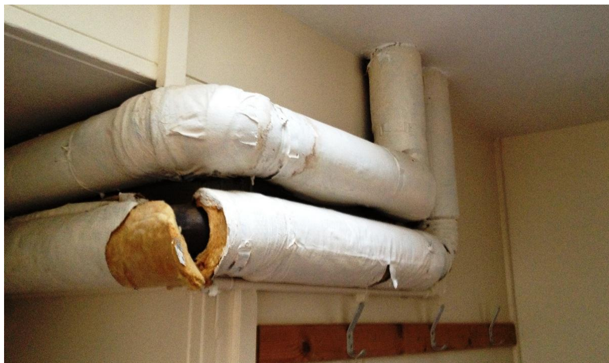
Figure 4: Existing flow & return pipes proposed location for linking to new heating pipes
